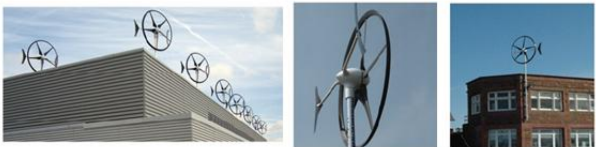
Figure 25: Swift Rooftop Wind Turbines 40
