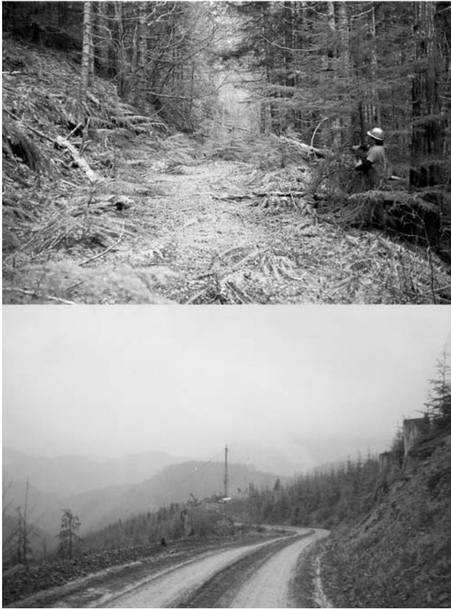
Figure 1. Minimizing road density while maximizing operational value results in the decommissioning of unused roads producing minimal sediment (upper photo) while maintaining heavily trafficked roads producing most of the sediment (lower photo).
