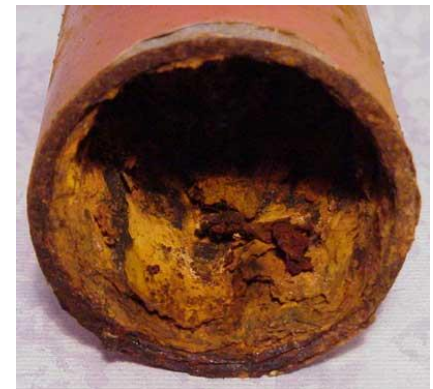
Rusty Pipe? CITY OF JGTON
