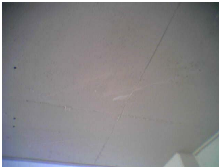
Figure 3: Cracks on the bottom of the same slab
