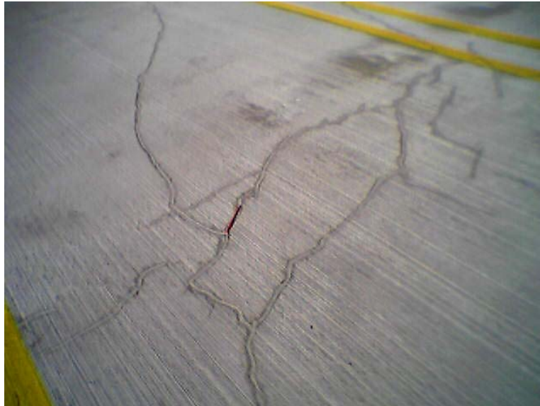
Figure 2: Cracks on the top floor of the parking structure
