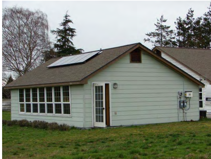
Figure 1. 1 kw (nominal, peak) solar PV system installed at EBLA
