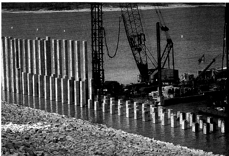
Figure 12.8 Compaction piles driven into the upstream embankment of Sardis Dam to reduce liquefaction hazards. The contractor drove the piles to this level with a barge-mounted conventional hammer; the piles were later driven below the water surface with a different hammer. (Photo by T. D. Stark; used with permission.)
