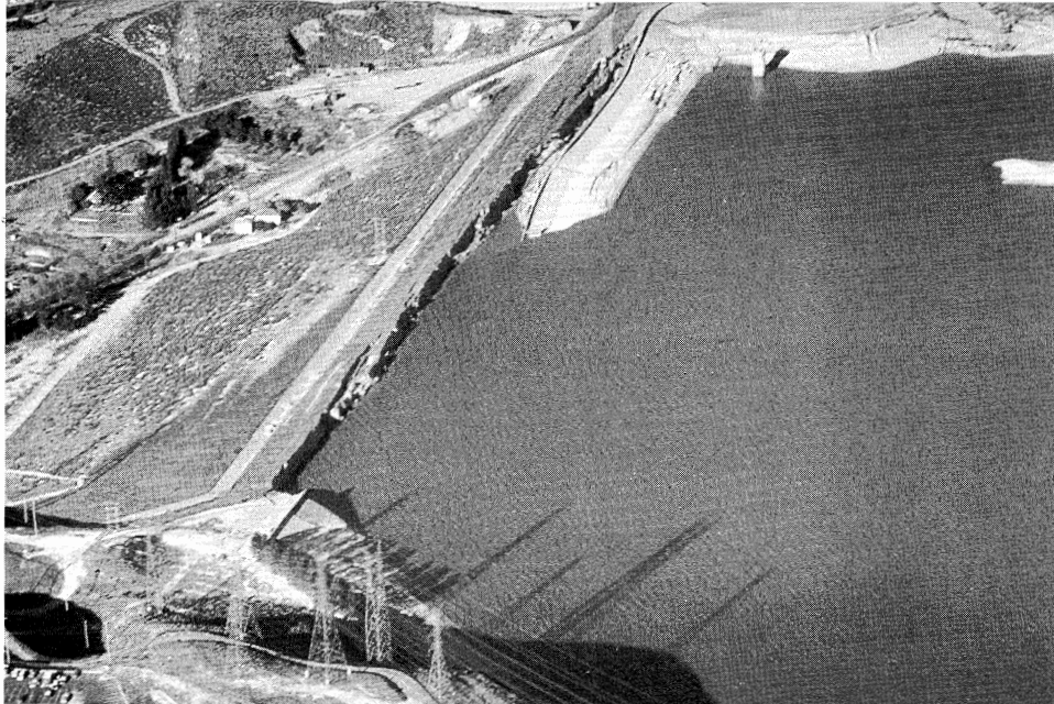
Figure 1.7 Lower San Fernando Dam following liquefaction failure of its upstream slope in the 1971 San Fernando earthquake (K. Steinbrugge collection; courtesy of EERC, Univ. of California).
