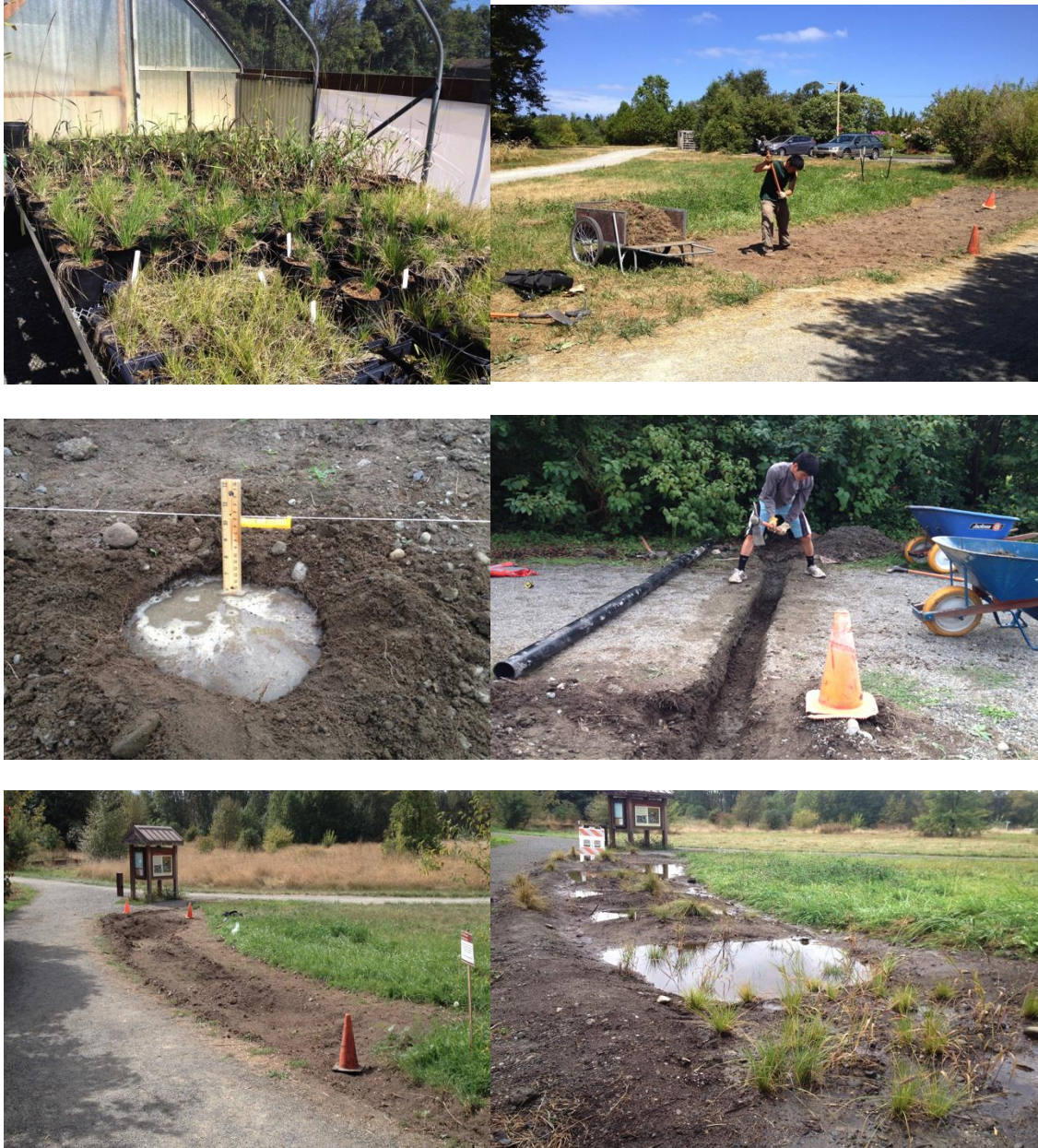
Figure 12: Installation photos. Clockwise from upper left: growing bunchgrasses in hoop house; removing sod; pipe installation, ponding after initial grading; initial grading and sod removal complete; infiltration test.
