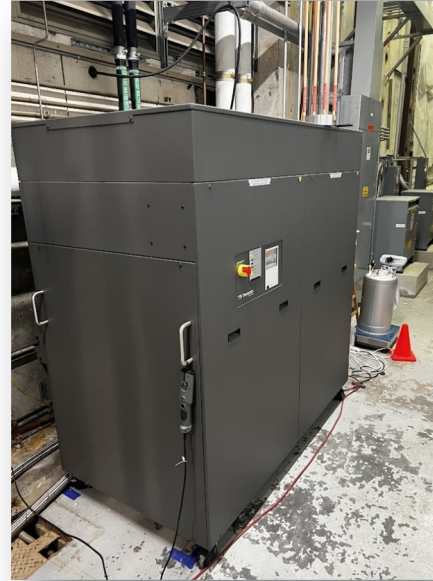
Chiller at SLAC with HFE-7100
