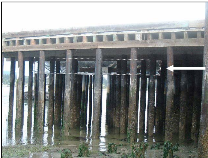
Figure IV.4. Reflective Panels (photo).
