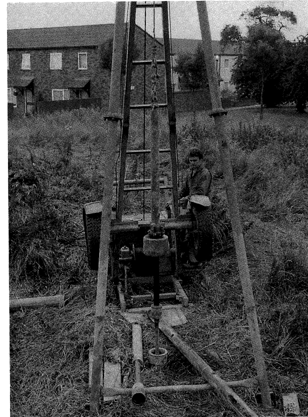
Light percussion rig sampling soils to a depth of 10 m for a construction project in Derbyshire
