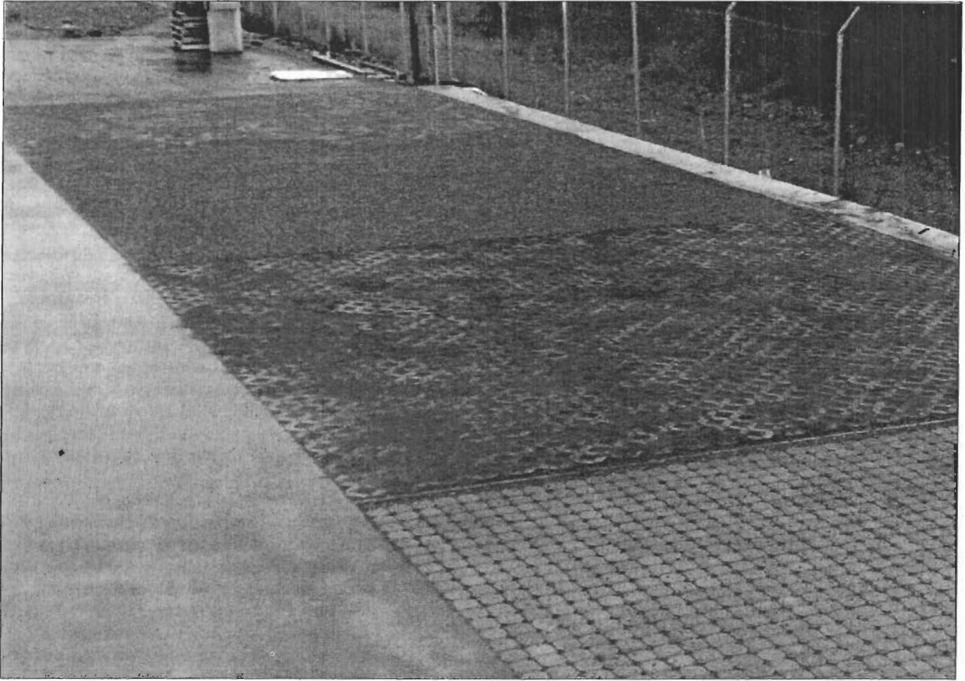
FIGURE 1. Test site shortly after construction and seeding (asphalt berm not yet installed).
